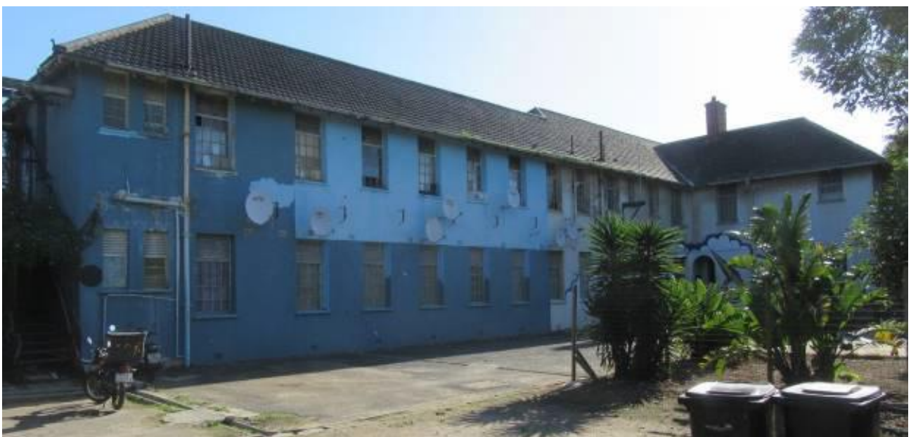
Photograph 4.10: Back (facing Alexandra Road) of Block D. As evidenced by the satellite dishes, the top storey is used for residential purposes.
