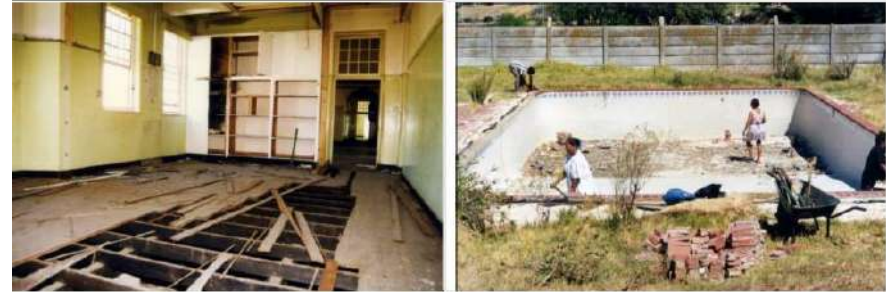
Figures 36 & Figure 37: Floors broken out in one of the F-shaped buildings, late-1990s/ early 2000s (left), and cleaning up the pool area, around 2001 (Source: Oude Molen Eco Village, 2013c).
