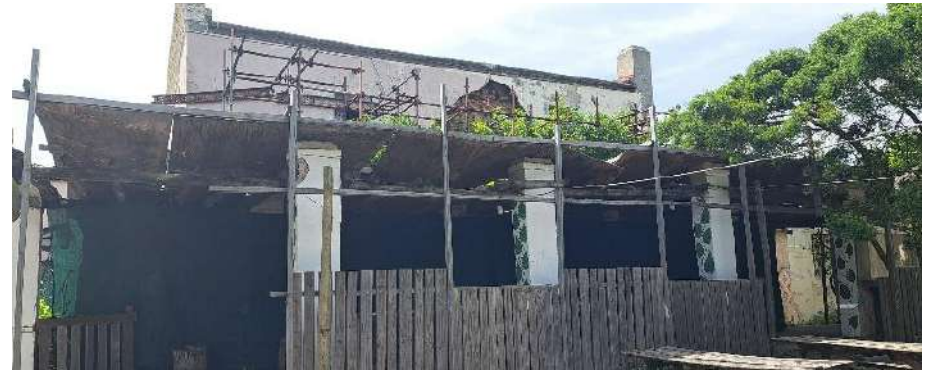
Figure 92: Homestead west elevation, screened by pergola (the latter likely remnants of an earlier mid-century building, subsequently burnt).
