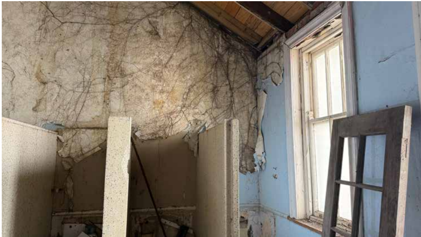
Figure 184. Plant and root ingrowth should be neutralised and removed to prevent further damage (RSA, April 2026)
