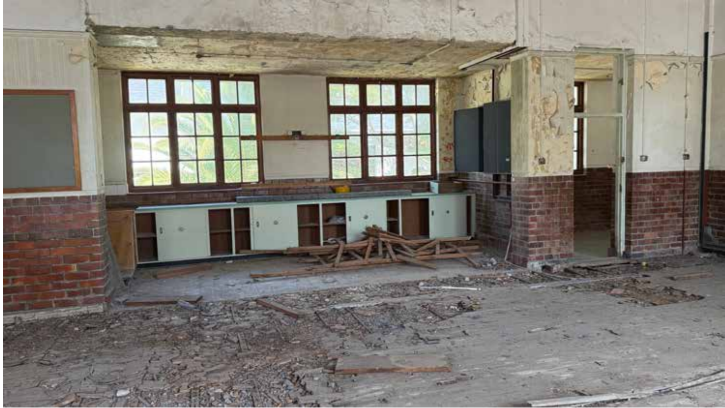
Figure 191. Damage and debris in classrooms to be cleaned up and the area safeguarded (RSA, April 2026)
