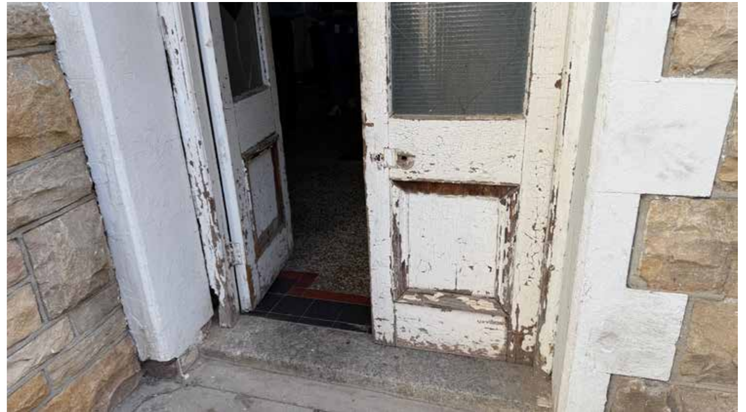
Figure 186. Historic joinery should be repaired and decorated and not left to further degrade (RSA, April 2026)
