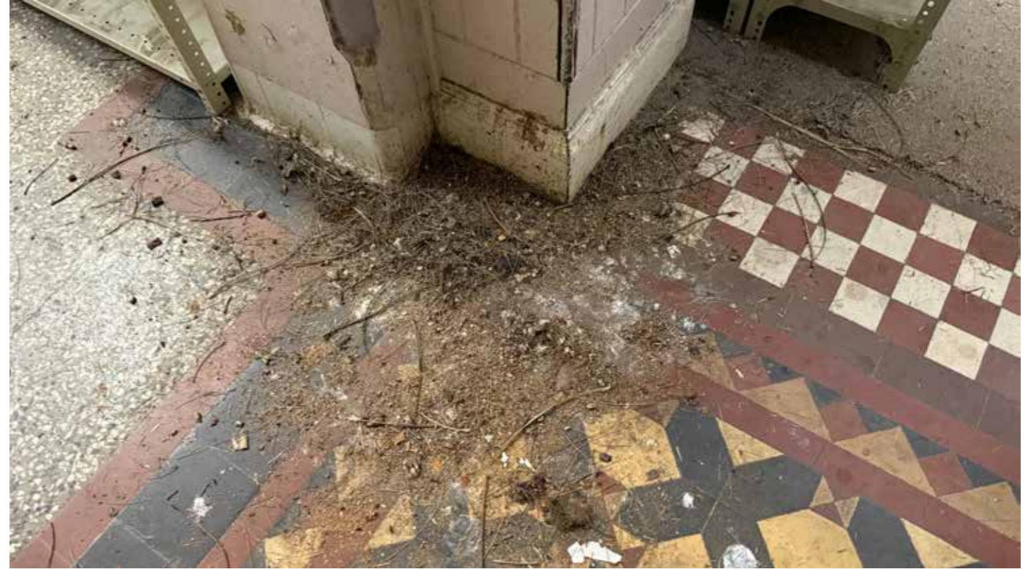
Figure 185. Birds and other wildlife should be kept out of the building (RSA, April 2026)
