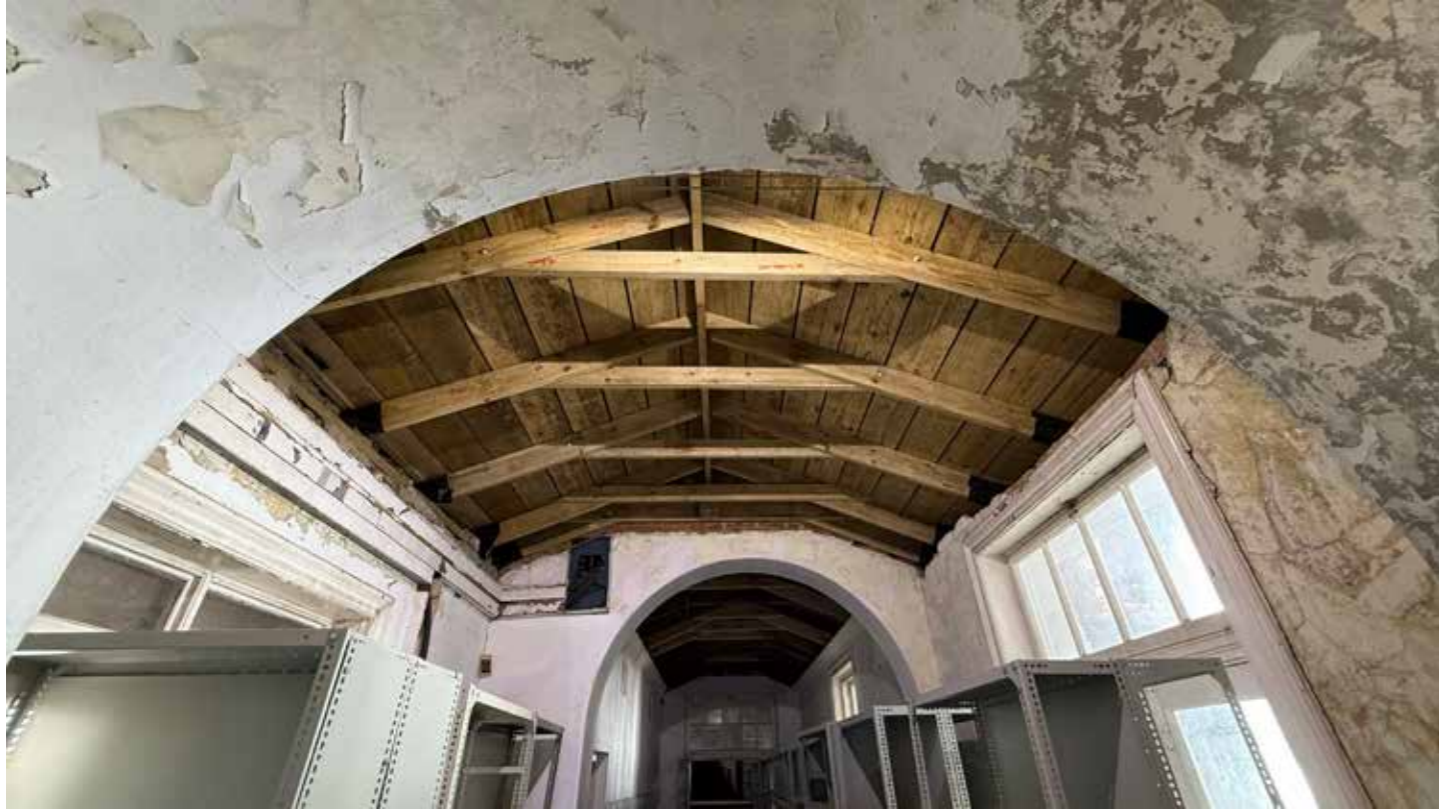
Figure 183. Areas already previously repaired and re-roofed should be recorded and monitored (RSA, April 2026)
