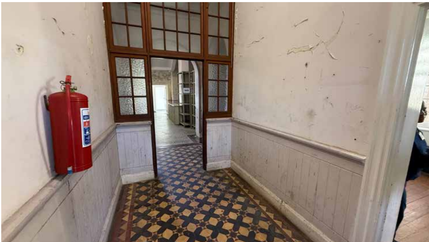
Figure 179. Fire protection and detection systems should be in place and operational (RSA, April 2026)
